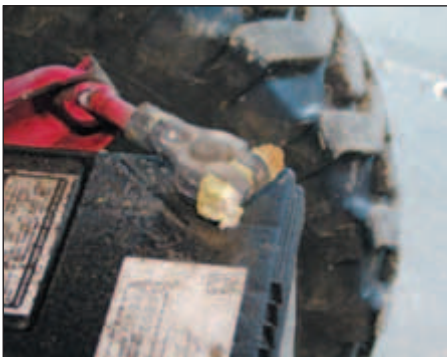
Bad battery – If the terminals are corroded, the circuit's voltage can drop and the charging system may not function properly.
