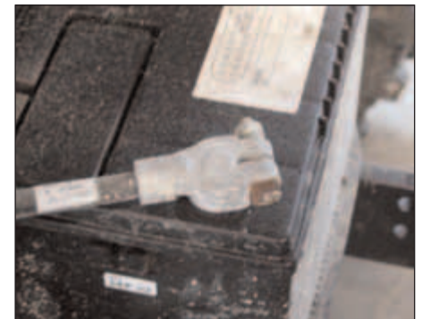
Good battery – Take the positive and negative (ground) cables off the battery and remove any corrosion from both of them.
